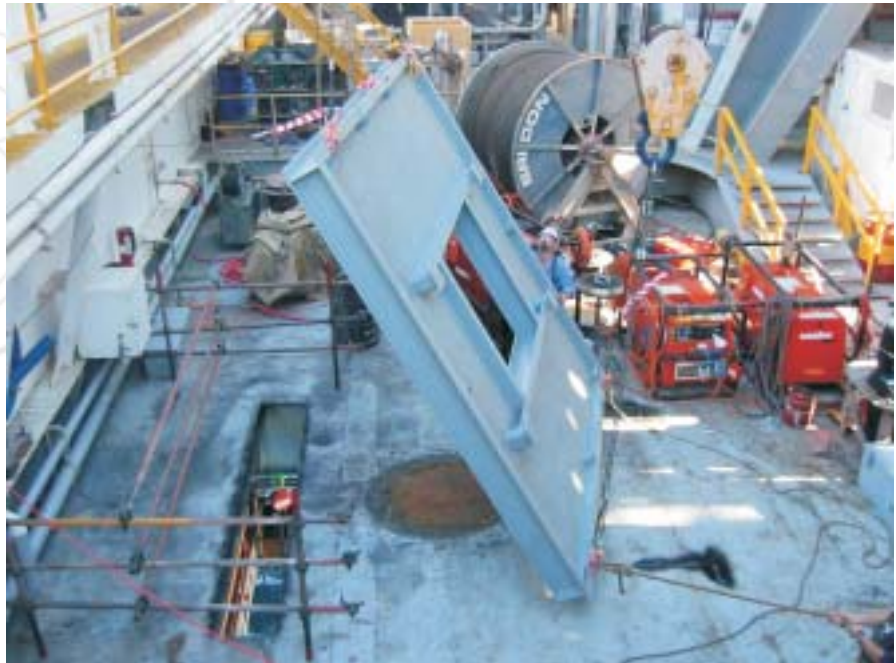
Retractable test stump platform ready to be lowered through the main deck.
