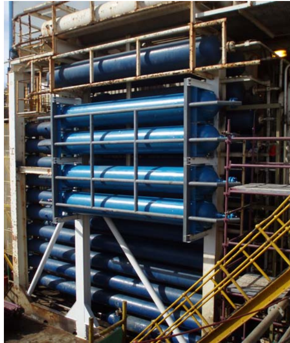
Modified APV Rack with additional 4 APVs installed
