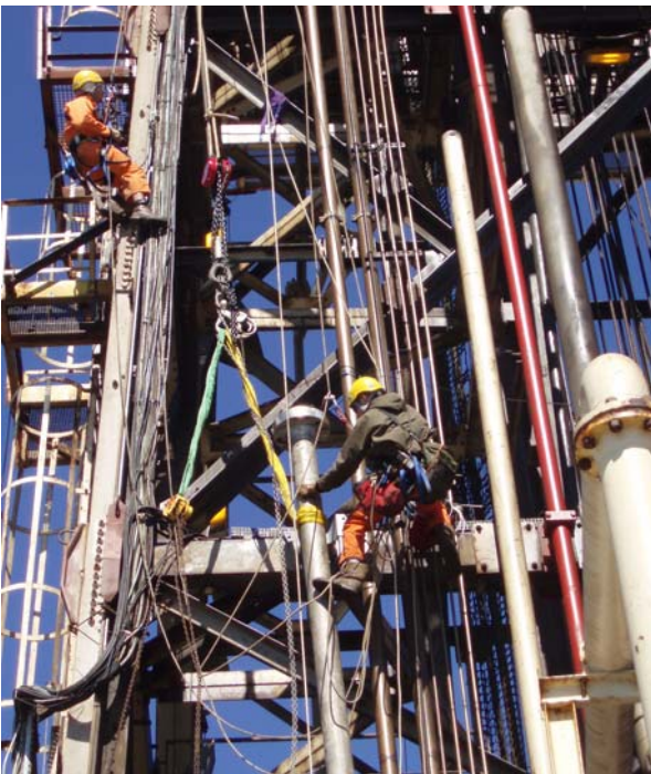
AME Rope Access technicians installing pipe supports and spools on the derrick
